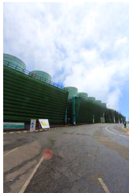
Fig.15 Huge geothermal power plant
