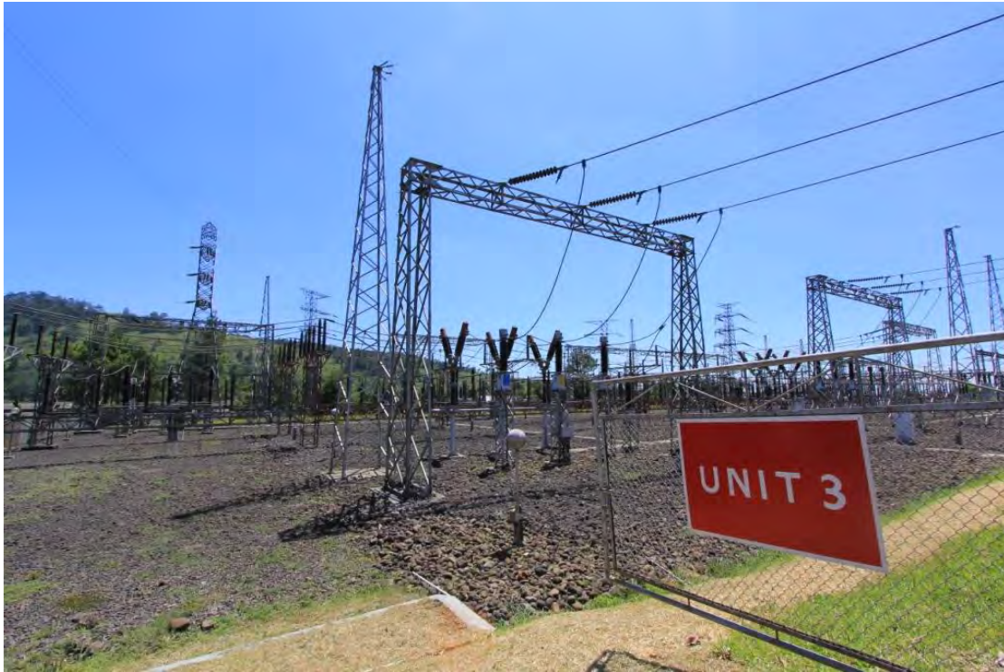
Fig.16 Huge geothermal power plant
